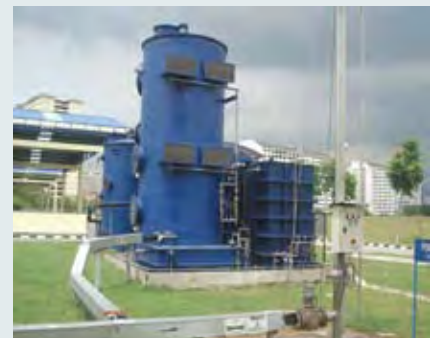
Effluent water reclamation for non-potable & industrial purposes
