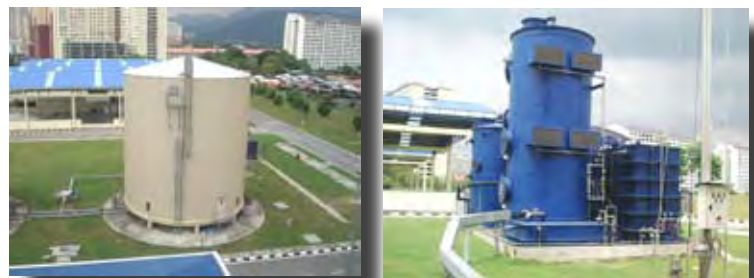
Biogas Engine for power generation
