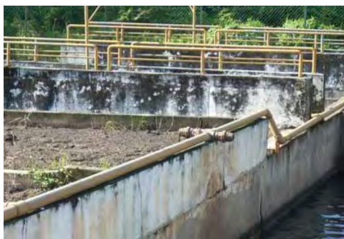
Stolen valve at drying bed
