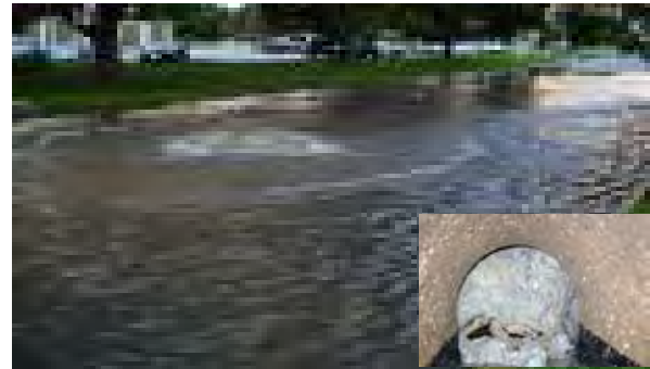
Overflow of sewage from manhole and major sewer blockage
